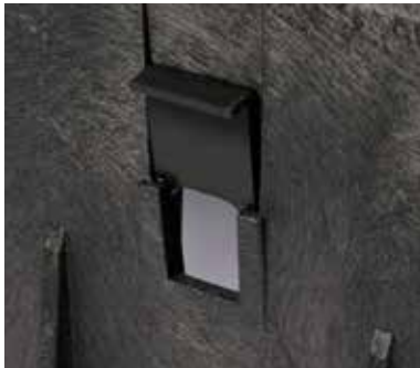
Temporary drop port
